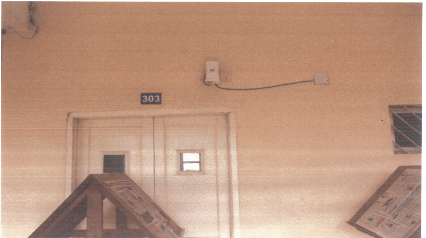
CAMPUS WI-FI ACCESS POINT -1
