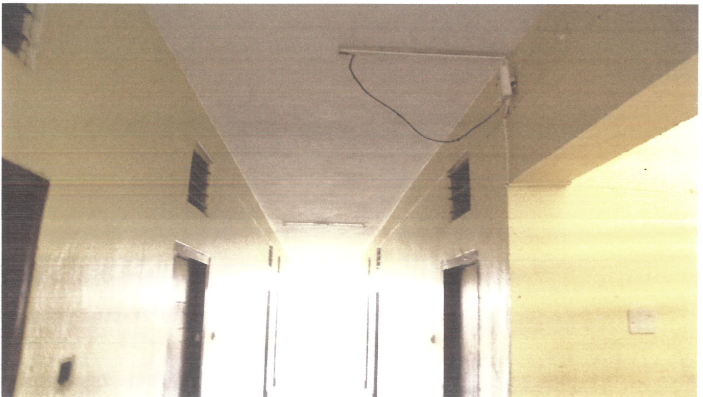
BOYS HOSTEL WI-FI ACCESS POINT -2
