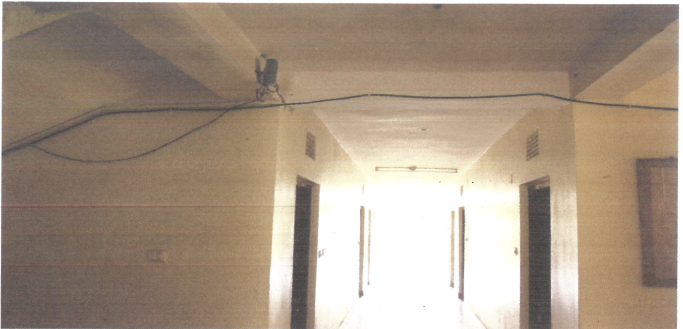
BOYS HOSTEL WI-FI ACCESS POINT-1
