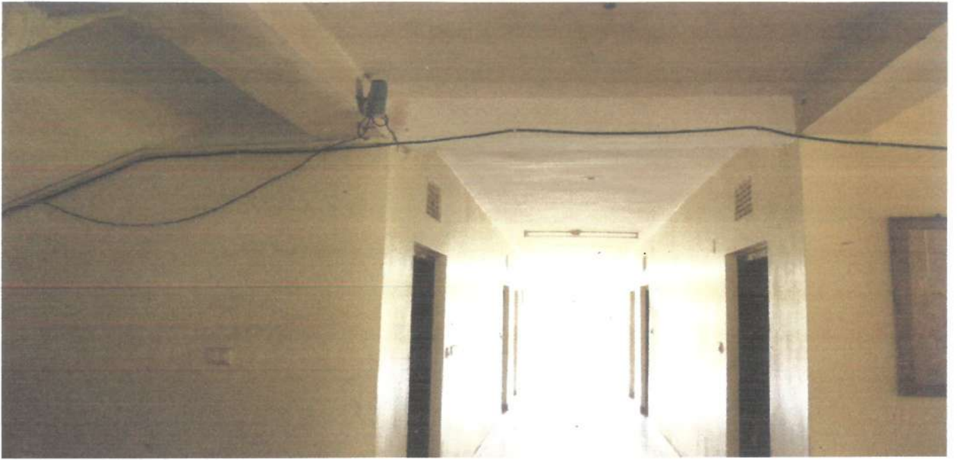
BOYS HOSTEL WI-FI ACCESS POINT-1
