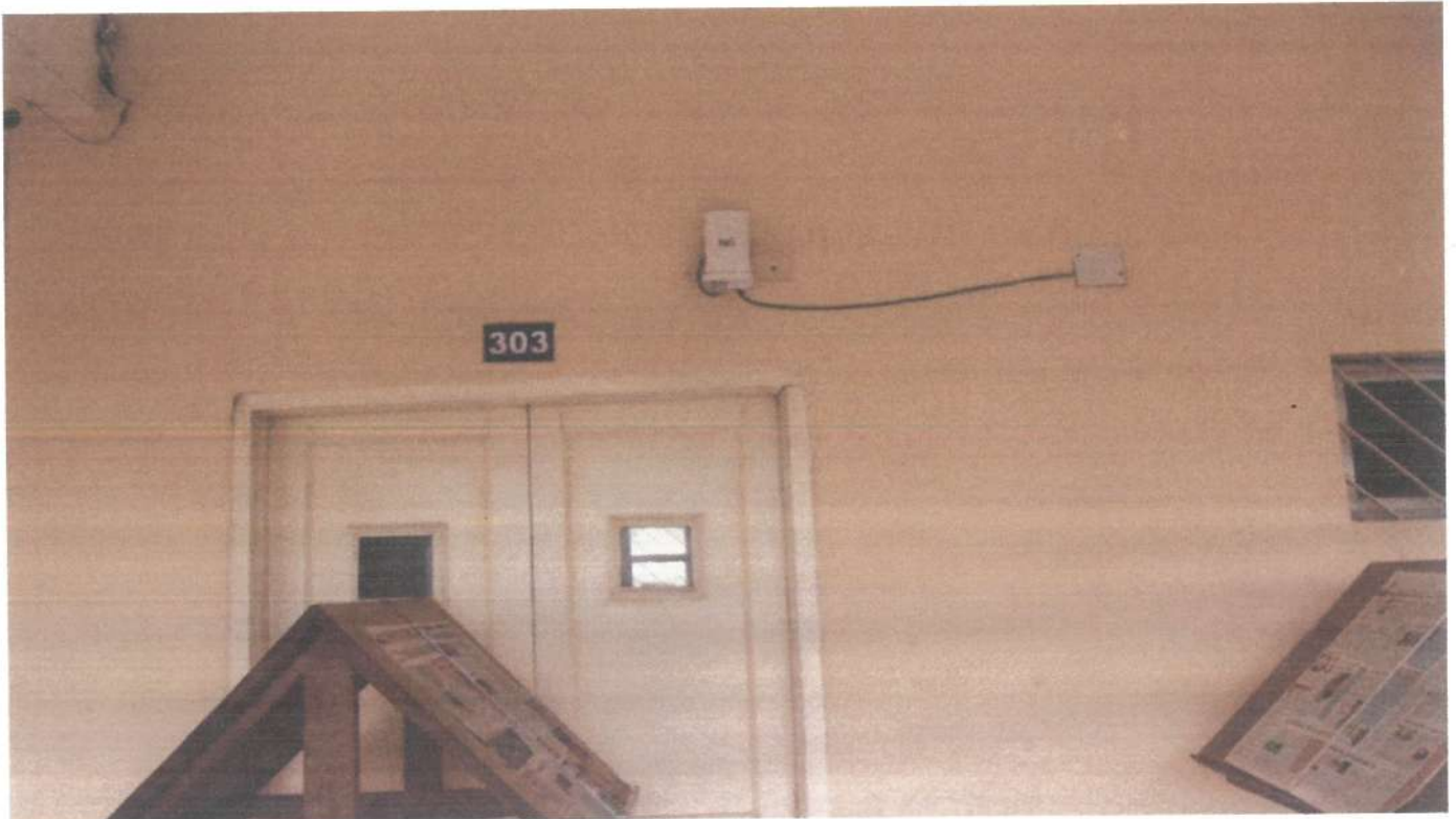
CAMPUS WI-FI ACCESS POINT -1
