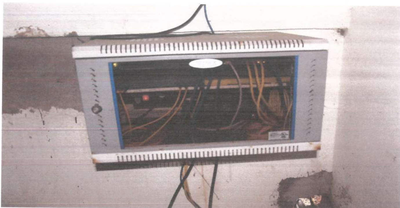
LADIES HOSTEL WI-FI ACCESS DISTRIBUTION SWITCH
