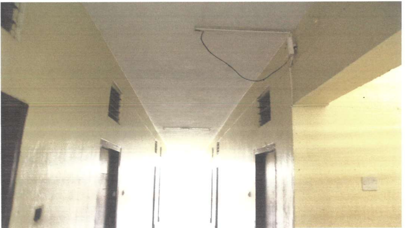
BOYS HOSTEL WI-FI ACCESS POINT -2
